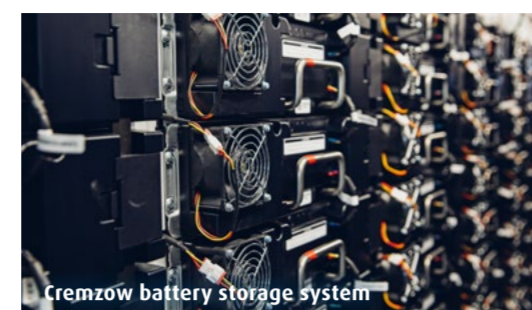
Cremzow battery storage system
