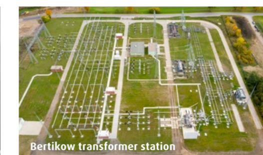
Bertikow transformer station
